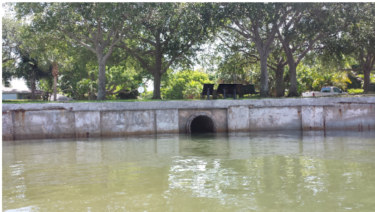
Discharge pipe at Sun Circle Park
